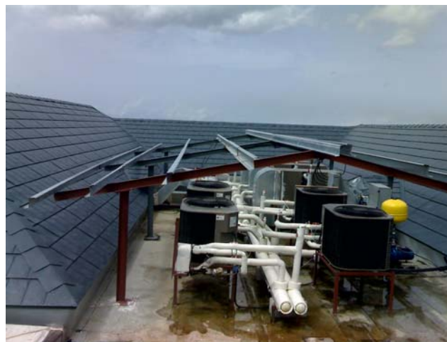
Fig. 5 – High Efficiency Mini Chiller with Heat Recovery
